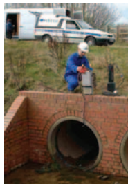
OnSite undertakes flow surveys for Severn Trent Water as part of its term contract agreement.
